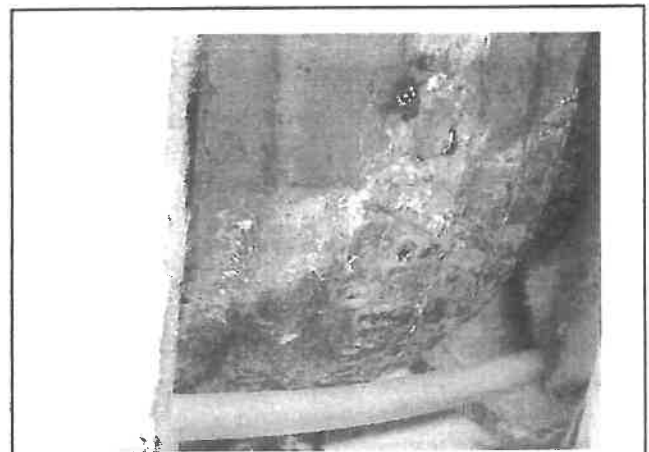
Corrosion and condensation in new Vancouver condominiums
